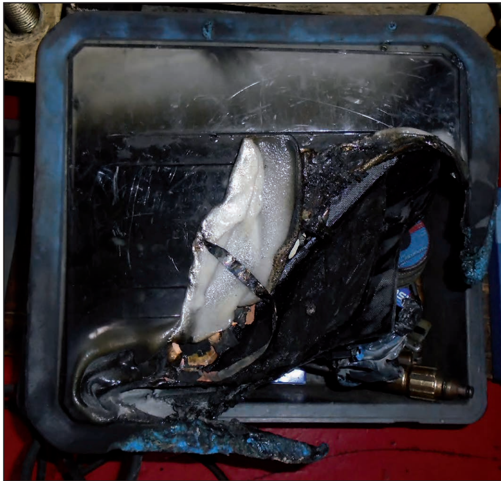
Figure 2: Damaged light unit
